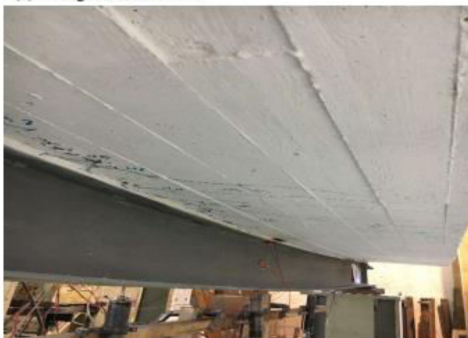
(b) Underside concrete cracks
