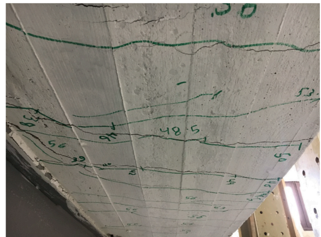
(a) Transverse cracks at the lower surface of the concrete slab
